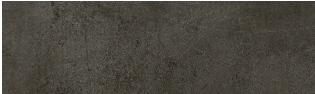
N NOT-3995 Scratched Concrete
