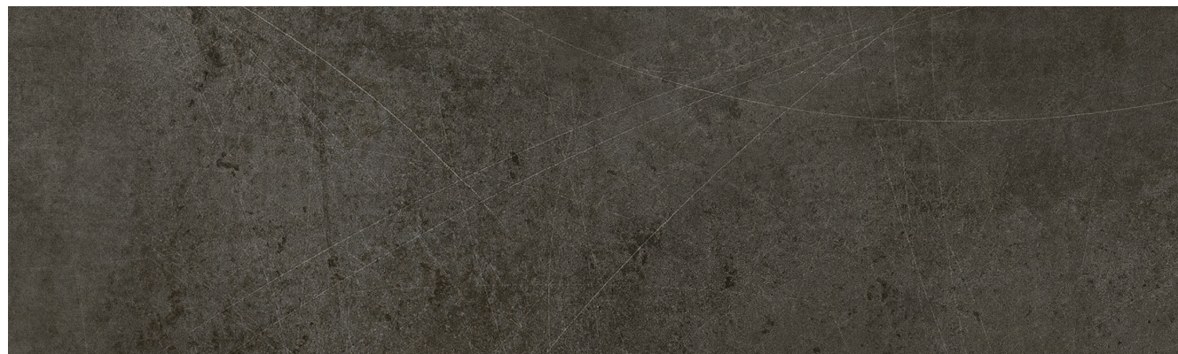
N NOT-3995 Scratched Concrete
